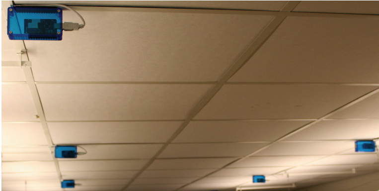
Figure 1.1: The picture shows a part of the wireless sensor network testbed mounted in the ceiling at the Automatic Control Lab at KTH; see Maciel (2008) for full details. Each box contains a Tmote Sky mote equipped with a temperature sensor, and a majority of the motes also have an ultrasound receiver. The motes communicate with each other using radios compliant with the IEEE 802.15.4 standard. The wiring that can be seen supplies power and is not used for communication.
